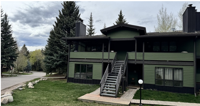
Building H, Par Six Condominiums. Recent exterior repaint and new metal siding.
